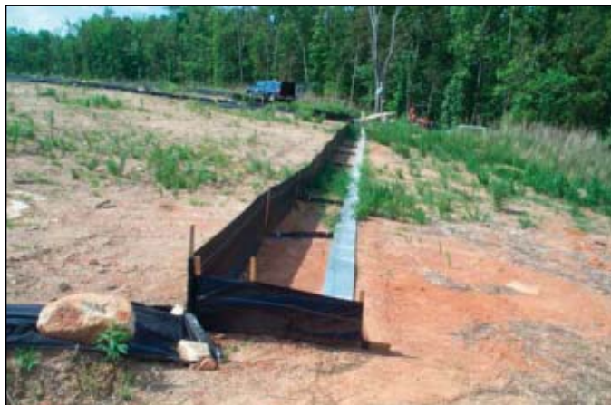
Installation of a conventional silt fence at the same landfill site provided a basis for comparison (Fig. 3).
