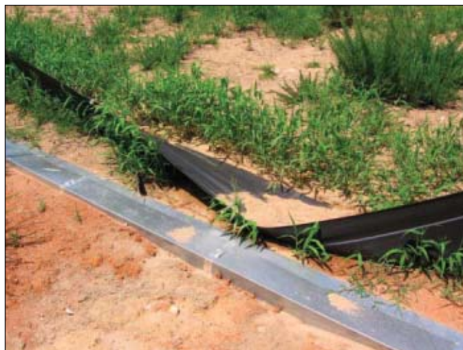
Storms between June 14 and July 5, 2007, damaged the conventional fence installed on the same site at which FAEST remained intact (Figs. 7-8).
