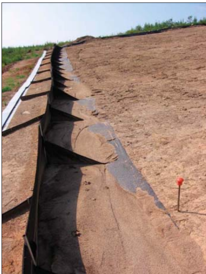
While trapping sediment, FAEST remained intact with all posts erect and no undercutting (Fig. 6).
