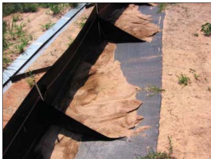
FAEST traps much more sediment, shown here, than the conventional fence (Fig. 5).
